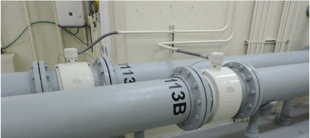
Photo of typical flow meter
