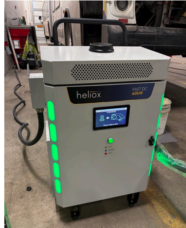
Heliox 60kW mobile maintenance charger
