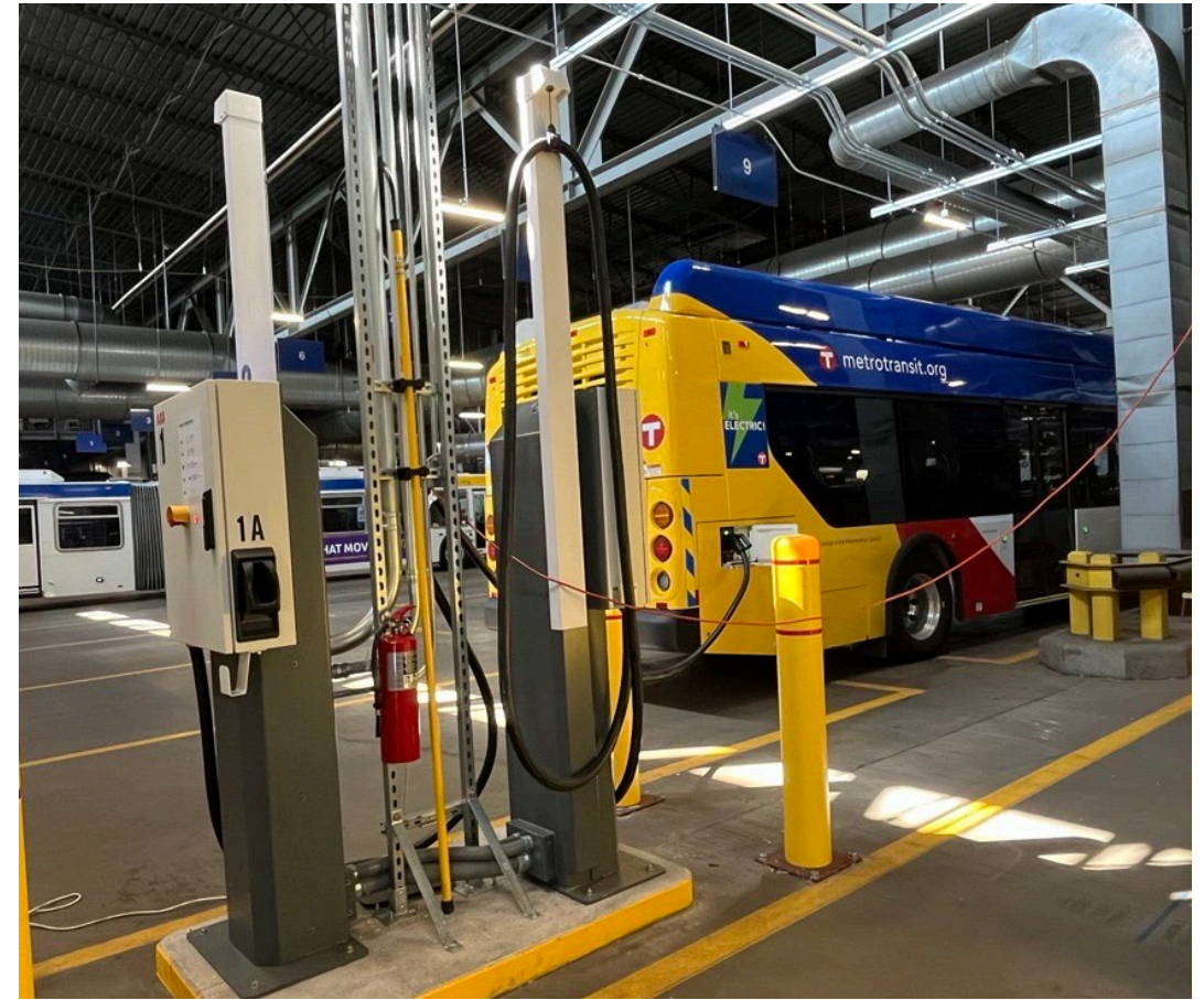
New flyer electric bus and ABB plug-in dispensers
