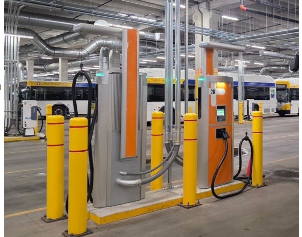
ChargePoint plug-in dispensers at North Loop Garage
